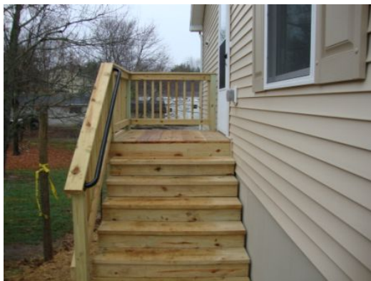
Handrail along guardrail
