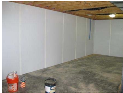
Fire rated insulation in basement
